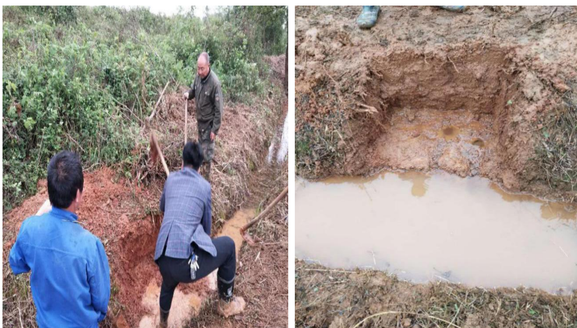
坝中段坝脚明显渗流
